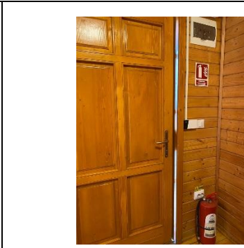
Fire extinguishers allocated based on fire department emergency plan
